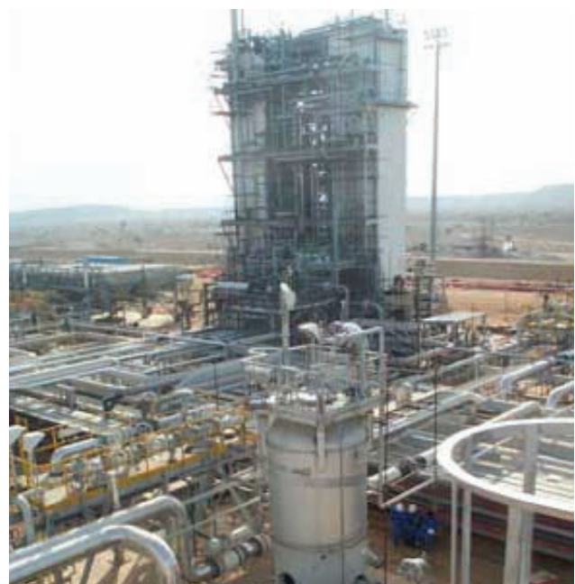
Mercury Removal Unit
