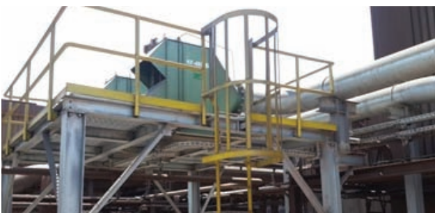
Inlet Air Filter
